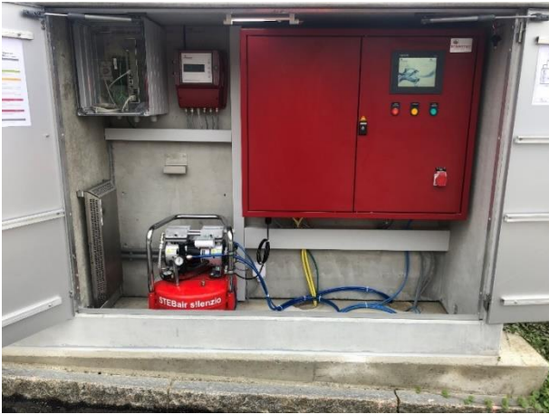
Figure 3: Cabin with STEBATEC control system, compressor and heating. The data connection via fibre optic cable to the DCS can be seen at the top left.
