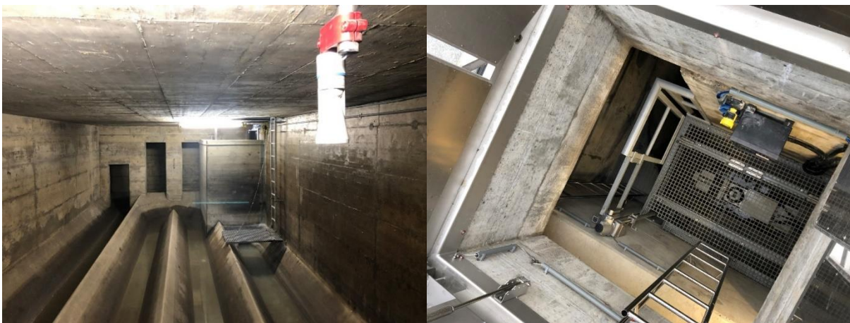
Figure 2 left: A shaft was built on the discharge side so that a pneumatic discharge controller could be used. In case of rain, the flow is reduced to use the volume of the basin. Right: The entrance to the throttle shaft, which is spacious and safe after the reconstruction.
