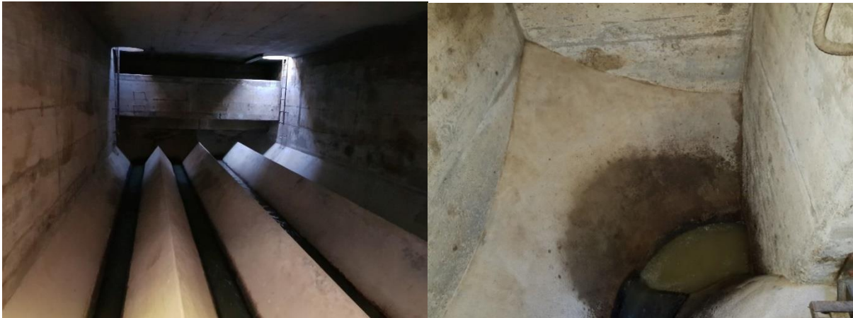
Figure 1: In dry weather the water flows zigzagging between the 'Toblerone structures'. In rainy weather and when the basin is filled, the water can be discharged in the discharge channel, visible at the left end of the pool. Right: Curve directly after the outlet of the Dätttau rainwater basin. After the curve, the pipe was not accessible, which is why a partition was newly built inside the basin to integrate the pneumatic discharge control.
